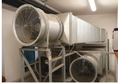
Figure 3: Staircase pressurisation fans on the top floor Source: compiled by the authors
