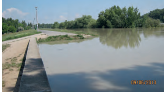
Figure 12. Earth dyke at the cross section change in Budapest, Pünkösdfürdő in the 2013 flood (Budapest Sewage Works Ltd.)
