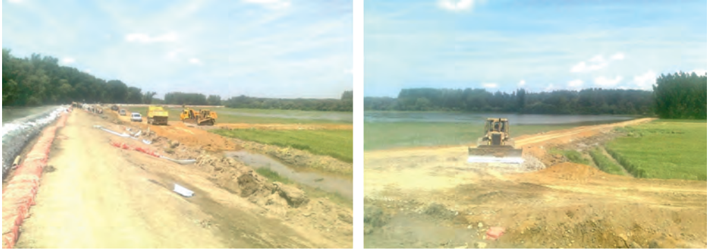
Figure 28–29. Flood protection road during the flood in 2013 in Győr (photo archive of NYUDUVIZIG)
