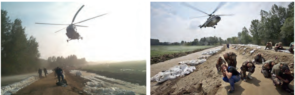
Figure 26–27. Placing sandbags by helicopter during the flood in 2013 in Győr (photo archive of NYUDUVIZIG)
