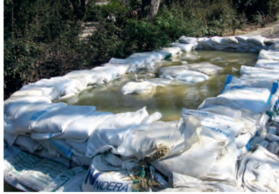
Figure 20. Counterpressure basin over a manhole, the overflow is not necessary in this case (Budapest Sewage Works Ltd.)
