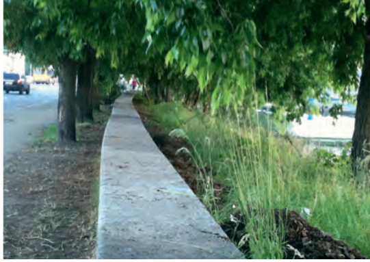
Figure 13. Low flood protection wall, Budapest (Budapest Sewage Works Ltd.)
