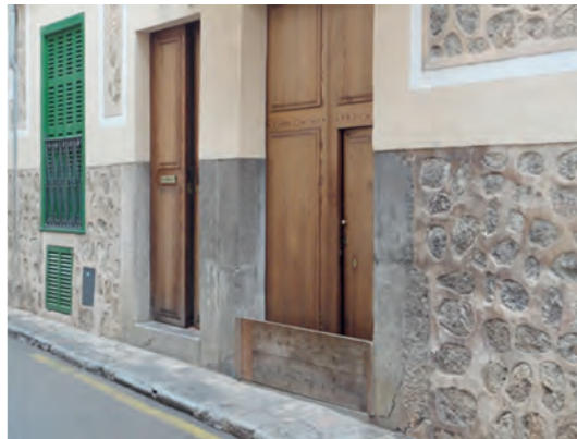
Figure 16. Elevated door sill and door flood barrier at Sóller in Mallorca (photo taken by the author)
