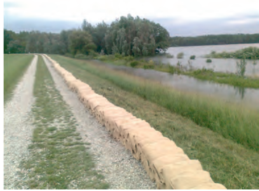
Figure 22. The correctly prepared protection line made of filled sandbags (photo archive of NYUDUVIZIG)
