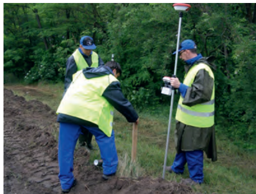
Figure 7. In case of heightening the levee, its height must also be marked (photo archive of NYUDUVIZIG)
