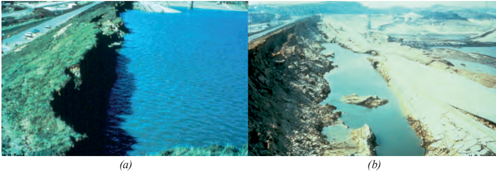
Figure 6. Lower San Fernando Dam, upstream face showing liquefaction slide due to earthquake (M 7.1) shaking, a) immediately following the earthquake; b) after the reservoir was drawn down [17]
