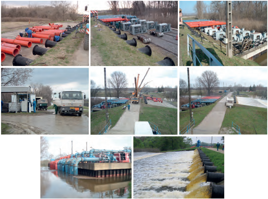
Figure 37. The temporary portable pump during the excess water control in the spring of 2013 (photo archives of TIVIZIG, KÖVIZIG and KÖTIVIZIG)
