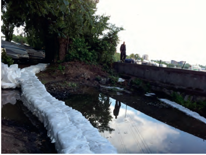
Figure 16. High flood protection wall, seepage control by counterpressure basin, Budapest, 2013 (Budapest Sewage Works Ltd.)
