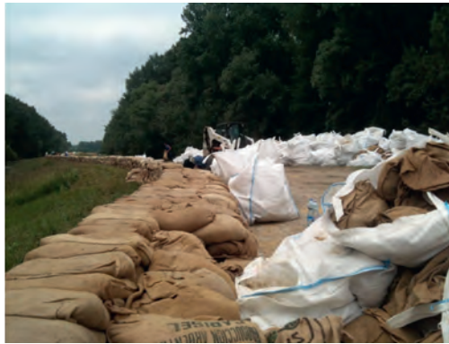
Figure 18. The most important material of flood protection is the sandbag (photo archive of NYUDUVIZIG)
