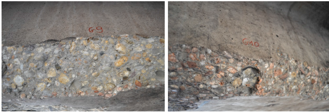
Fig. 12. Surface of the spalled concrete and the broken aggregate grains. (12.07.2017).
