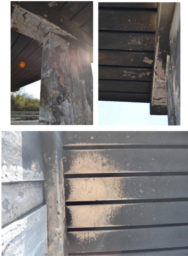
Fig. 4. Header and main beams after the fire (31/3/2017).
