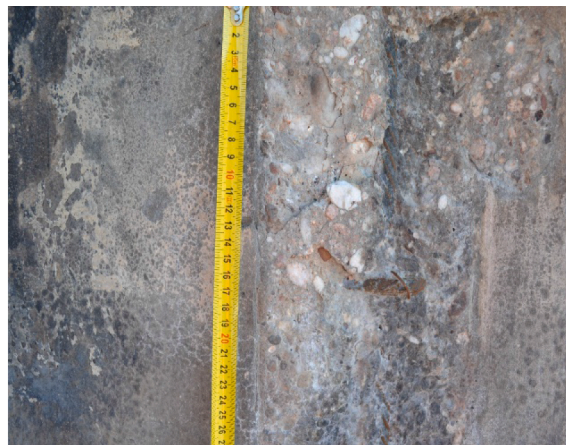
The spalled and discoloured concrete
