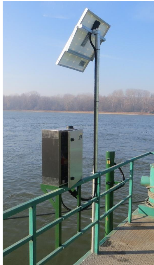
Figure 3. Automatic turbidity monitoring station (Danube, 1479.6 rkm, left bank, authors' photo).
