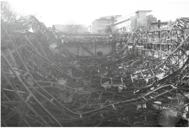
Fig. 4 The steel-roof structure after fire (15.10. 2015)
