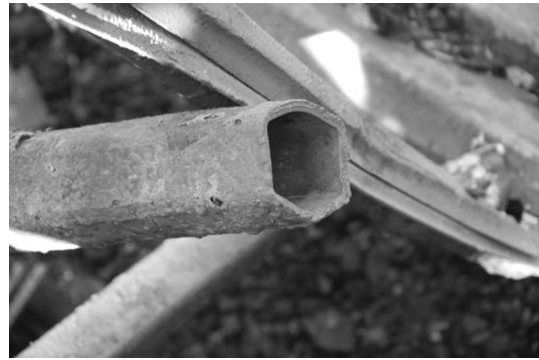
Fig. 6 Failure of welds (15.10. 2015)
