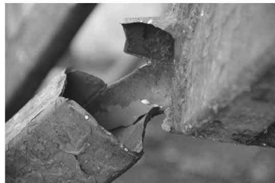
Fig. 7 Failure of weld and steel material (15.10. 2015)
