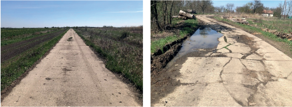
Figure 9. A concrete road in good and damaged condition (periphery of Besenyszög).
