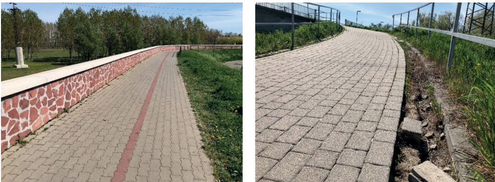
Figure 10. Paving-block surface in good and damaged condition (in Szolnok).
