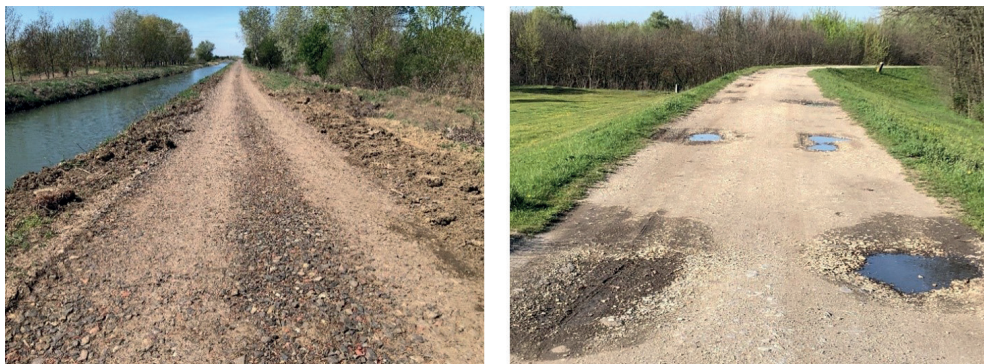
Figure 11. Gravel road in good condition and with damaged surface (periphery of Tiszasüly and Szolnok).
