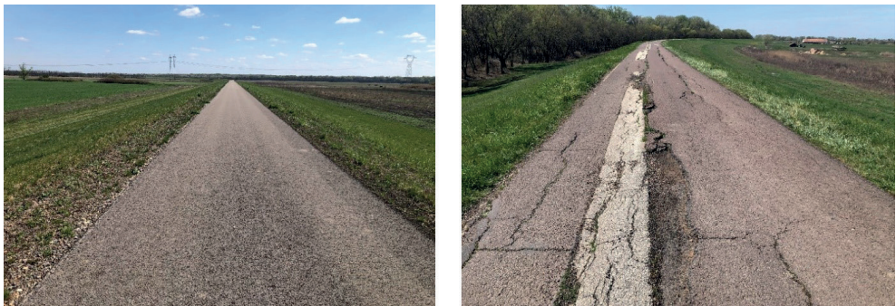
Figure 8. A tarmac road in good and damaged condition (periphery of Besenyszög and Pély)
