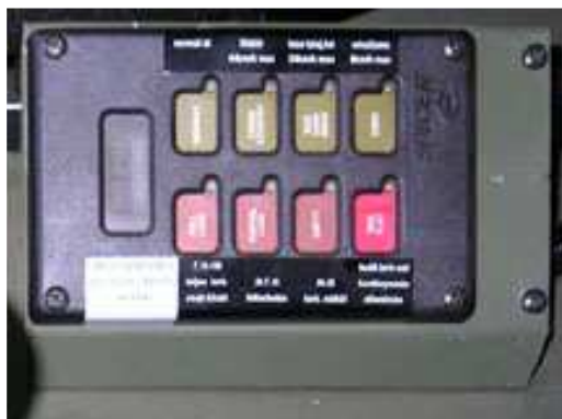
Fig.: 4.9 ábra. Control station with the selecting switches
